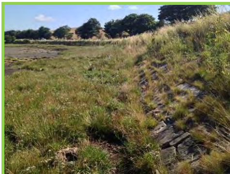
Gaps between blocks and overgrowth on stone revetment along B1342 (/1501c04).
