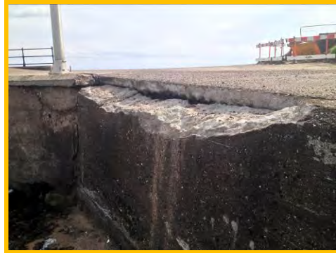
Localised spalling of the coping at the seaward end (/300c10).
