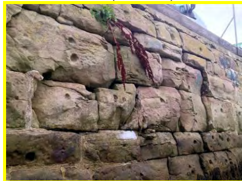
Apparent movement in an area of masonry blocks on outer face of Pier (/1701c14).
