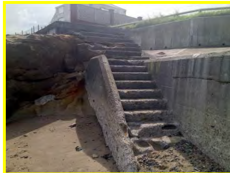
Highly abraded access steps presenting a public safety hazard (/3101c03).
