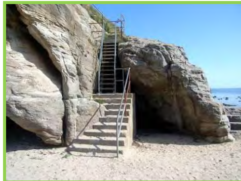
Deep caves adjacent to base of access steps (/701c05).
