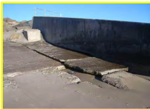
Undermining, settlement and cracking of to Hadston Scaurs outfall apron in 2012.
