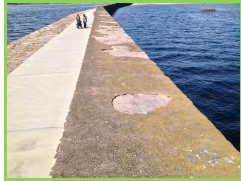
Spalling of concrete render on wave wall (/701c14).
