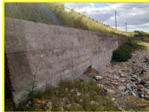
Masonry and concrete seawalls north of Dell Point in fair condition (/1701c25).
