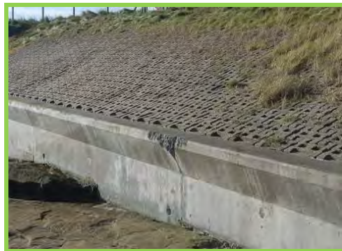
Minor abrasion to low concrete wall at south end of Cresswell (/3201c19).
