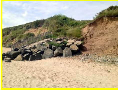
Rock armour at access steps in fair condition but outflanking continues (/2601c09).
