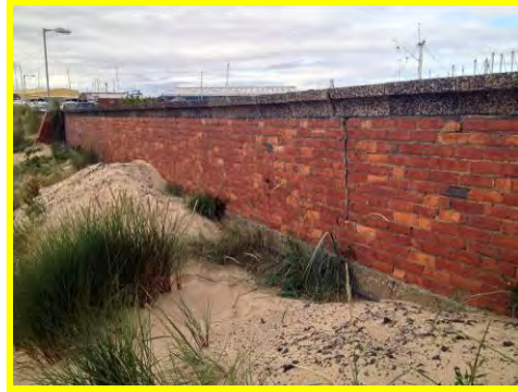
Some vertical cracking in the brickwork and loss of mortar at the coping (/4201c10).
