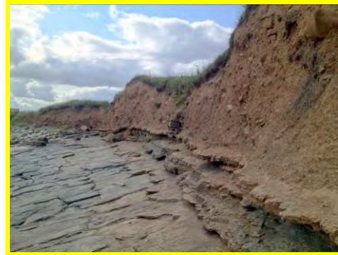
Erosion of the thin earth ridge (2m wide) at North Sunderland Point (/1701c23).
