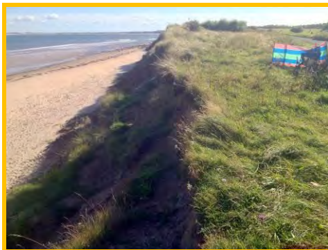
Active erosion of low earth cliffs and dunes in northern extent of Druridge Bay (/3201c14).
