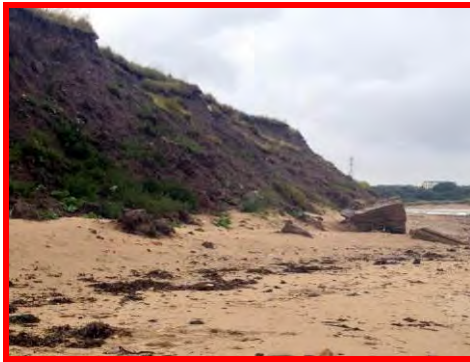
Continued slumps along the cliffs and breakup of pill box at Cambois House (/3901c01).
