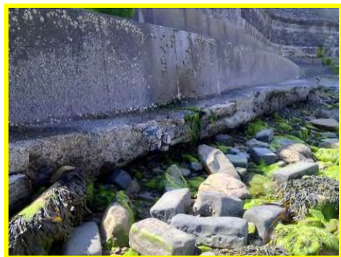
Abrasion, rotting timber wailing and undercutting at toe of seawall (/4401c16).
