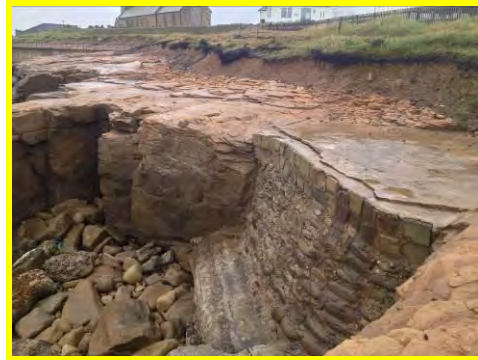
Abrasion and undermining of toe of localised masonry/ concrete walls (3601c01).
