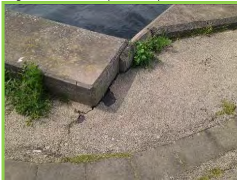
Crack in surfacing behind short section of masonry blockwork (/801c03).
