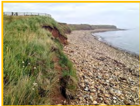
Recent erosion of earth cliffs at Red Brae in 2014 (/5001c05).
