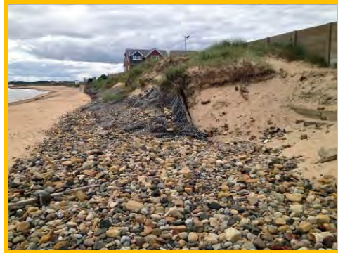
Outflanking of gabions at north end, erosion of dunes and exposure of wall foundations (/4201c03).
