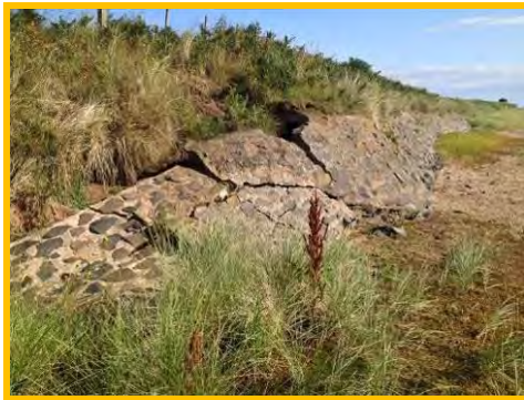
Undermining and collapse of south end of grouted stone revetment at Links End (/1401c27).
