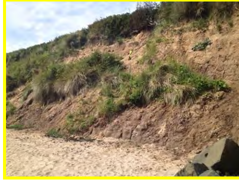
Signs of significant historic slippage along the cliffs south of Seaton Point (/2601c09).
