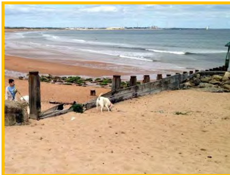
Missing planks and damage to timber groyne at mouth of Seaton Burn (/4402c02).
