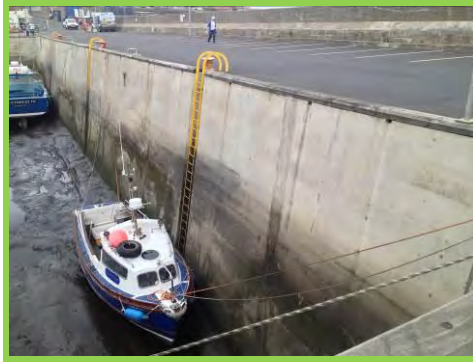
Inner face of Main Pier in good condition with only minor vertical cracks apparent (/1701c11).
