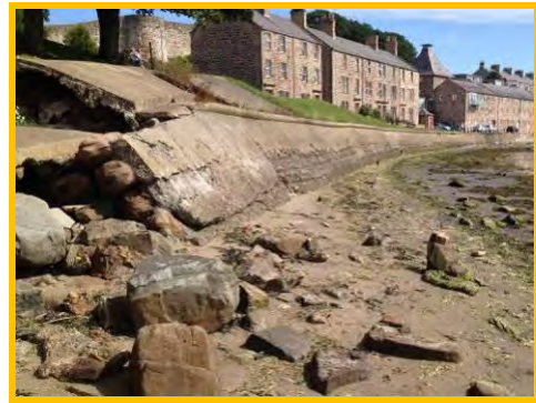
Outflanking and collapse at the south end of seawall (/801c07).
