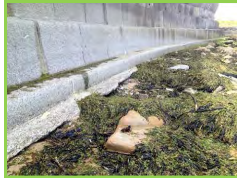
Initial undermining of toe at north end of wall (/4401c08).
