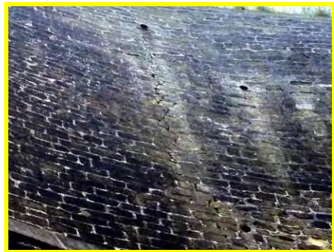
Full height gaps in the brickwork in the upper wall (/4401c15).
