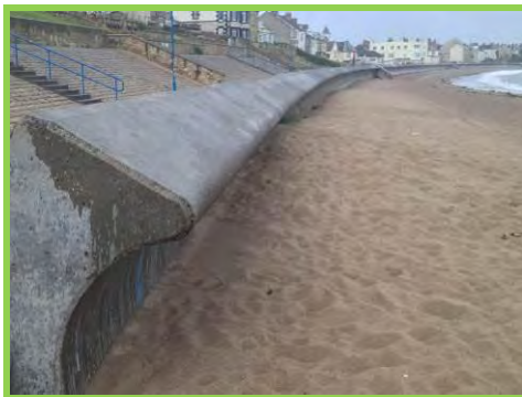
Increased beach levels largely burying toe apron of Newbiggin seawall (/3601c07).
