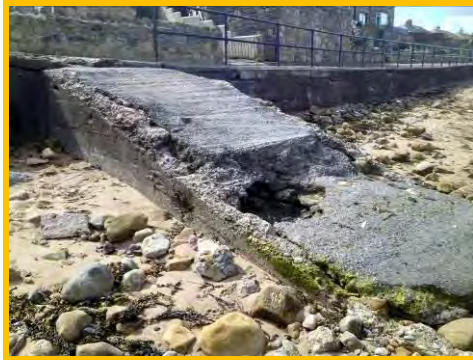
Abrasion, spalling and voids in seawall access ramp (/300c10).
