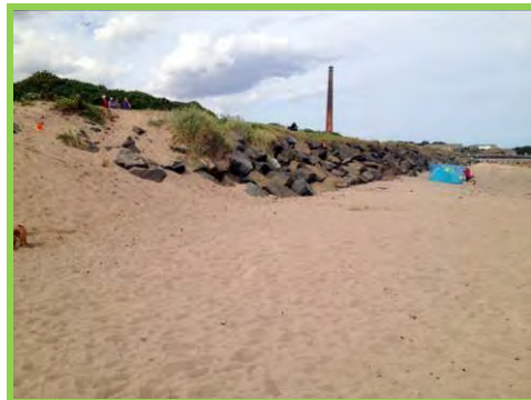
High beach levels burying south end of revetment (/1001c01).
