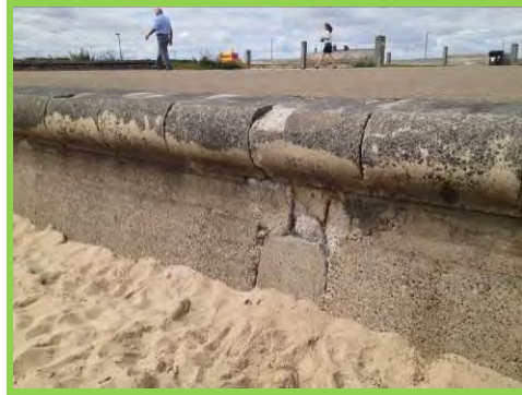
High beach levels, minor cracks and gaps at construction joints (/4201c07).
