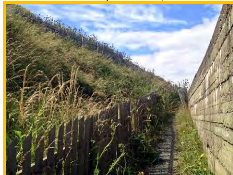
Movement in fencing along the access path above the high seawall.
