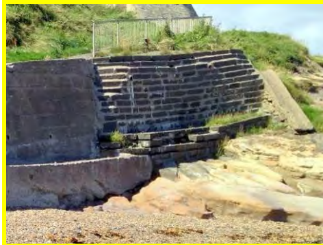
Missing bricks along toe of wall supporting access ramp (/4401c17).
