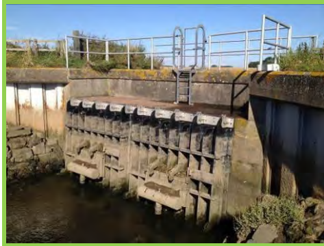
The sluice structure south of Ross Low channel appears in good condition (/1401c18).
