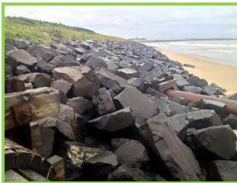
Some displaced rocks along toe of revetment fronting site of old foundry (/3901c05).
