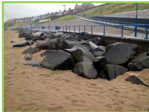
Rock armour largely buried by high beach levels at the south end of the bay (/3601c08).
