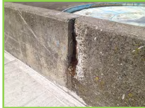
Spalling and rust staining to the setback wall, new concrete decking (/3101c05).
