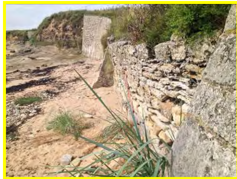
Weathering of blocks, missing mortar and seaward rotation of masonry retaining walls at Howick Haven (2501c01).
