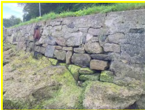
Gaps in the low masonry wall south along Dock Road (/901C05).
