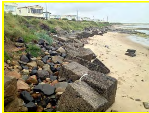
Cliffs fronting central section of caravan park stabilised by anti-tank blocks (/3501C06).
