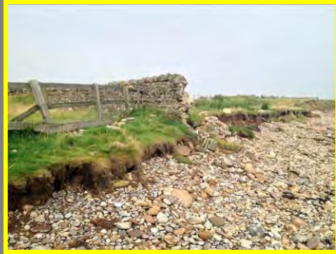
Erosion and partial collapse of boundary wall in 2014 (/4901c14).
