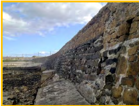
Masonry seawalls around Nackers Bay in poor condition (/1701c36).
