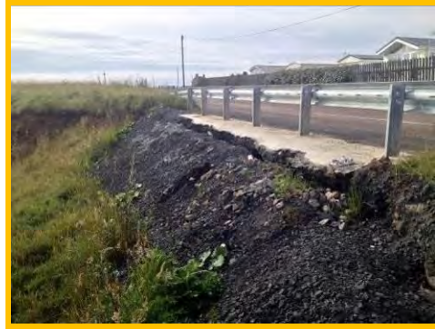
Slope showing recent signs of movement below the new barrier (3201c22).
