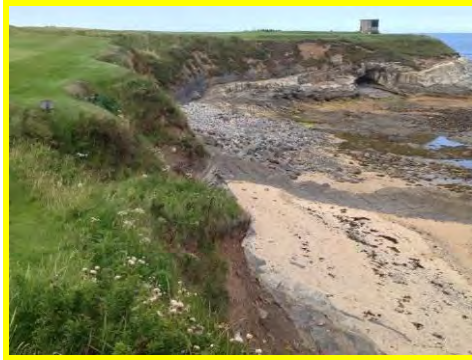
Erosion and cliffing of low earth cliffs fronting golf course (/1701c22).
