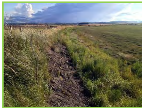
Asphalt and stone revetment largely overgrown (1401c98).
