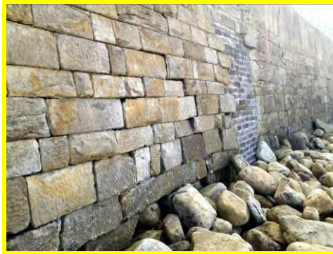
Cracks in upper section of masonry seawall on Rocky Island (/4401c11).
