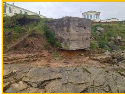
Pill box perched precariously on cliff edge (/3501C07).
