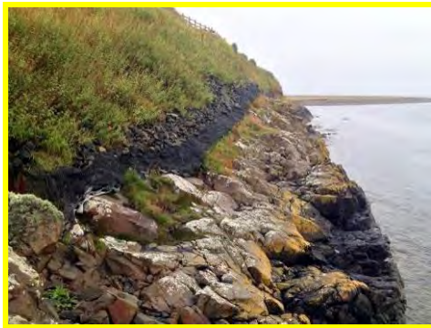
Hexagonal erosion control matting below castle in fair condition (/4901c12).
