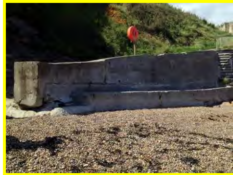
Large horizontal crack at base of wall and undercutting at south end (/4401c17).
