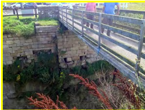
Gaps and missing blocks in the masonry wall along the man-made channel (/4401c07).
