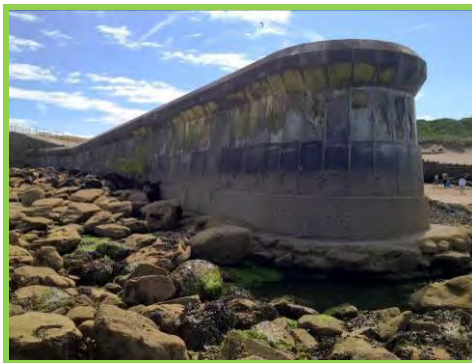
Undermining of toe at seaward end of pier (/4401c10).
