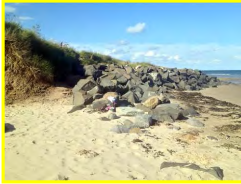
Outflanking of the revetment south of the Hadston Scaurs slipway (/3201c13).
