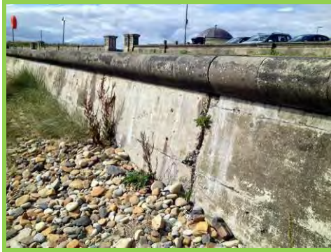
Minor cracks and spalling in the seawall to the south of the access ramp (/4201c05).
