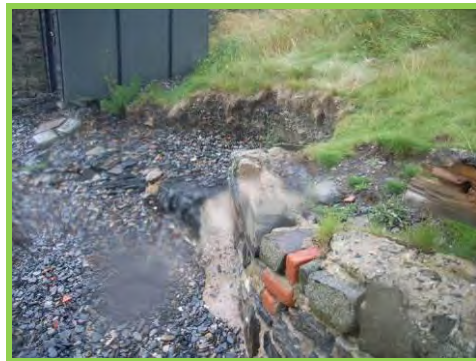
Lowering of beach levels at west end of masonry wall exposing previous outflanking (/4901c05).
