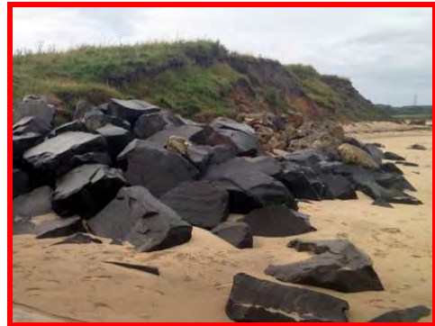
Rock armour and dumped concrete rubble partially stabilising cliff at slipway (/3901c01).
