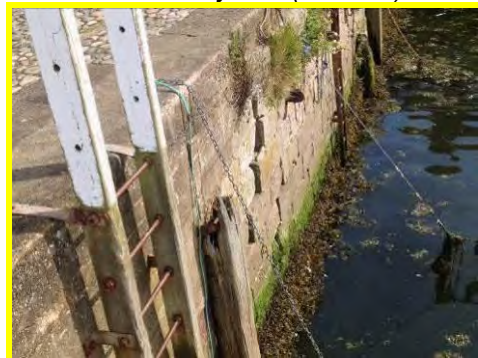
Vertical crack and potential movement of blocks in the north wall of the dock (/801c03).
