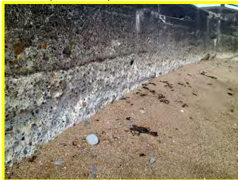
Horizontal cracks along South Pier and highly abraded toe (/3101c03).
