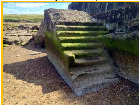
Significant abrasion of access steps from foreshore.
