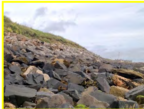
Dumped construction waste and smaller tipped rocks along crest (/4001c02).
