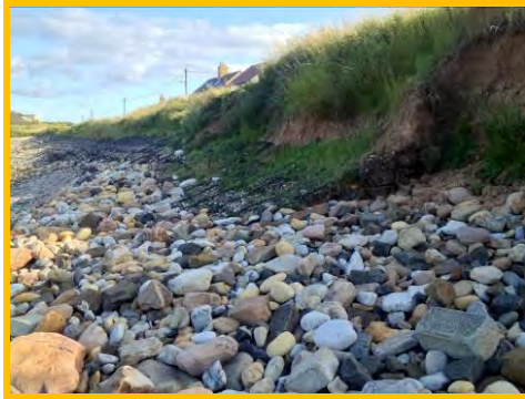
Burst baskets along the toe of the gabion revetment at Ladies Hole (/1701c39).
