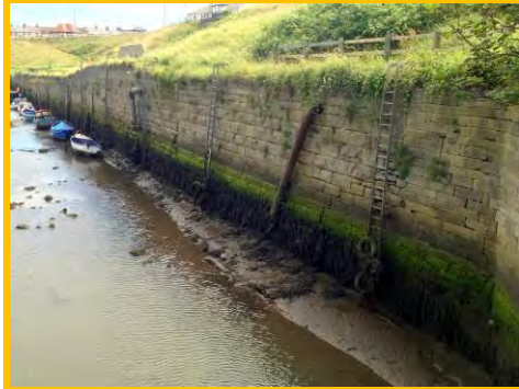
Gaps between blocks at west end of south bank quay wall (/4401c06).
