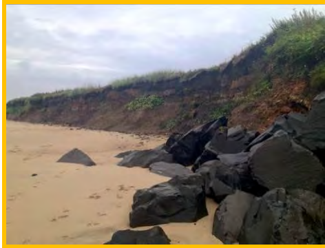
Erosion of earth cliffs and outflanking of revetment at south end (/3901c03).
