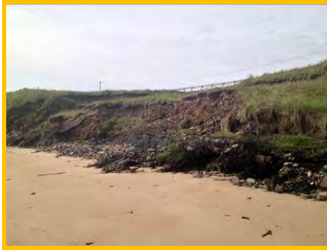
Damage to gabions and loss of material along toe of slopes north of Snab Point (3201c22).
