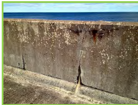
Minor cracking and missing joint sealant (/4401c10).
