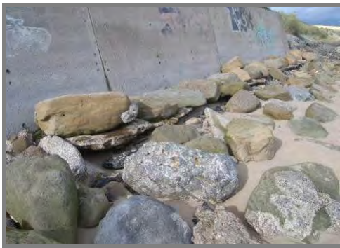
Low beach levels and undermining of toe of seawall in 2012.
