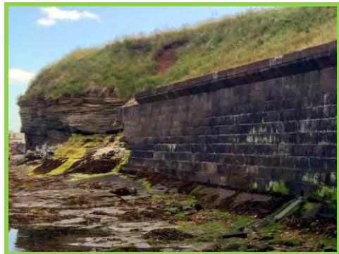
Erosion of upper earth cliff at east end of seawall.
