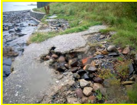
Damage to concrete apron along crest of wall (/4601c06).
