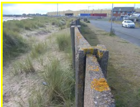
Some rotation of concrete post and plank wall at back of dunes (/4201c11).
