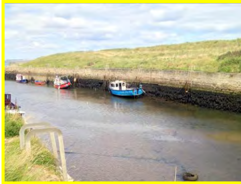
Missing mortar and gaps between blocks along eastern harbour quay wall (/4401c08).
