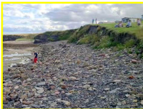
Erosion and cliffing of low earth cliffs fronting caravan park at Seahouse Pt (/1701c19).
