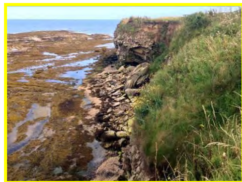
Localised rock falls near the sewage works at North Sunderland Point (/1701c22).
