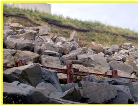
Corrosion and failed steelwork and slumps in upper earth slopes (/4001c02).
