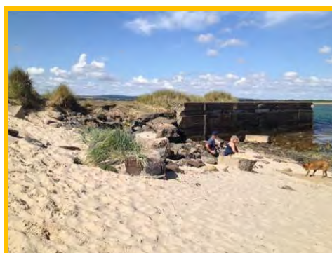
Partial collapse of northern wall of pier and loss of fill.
