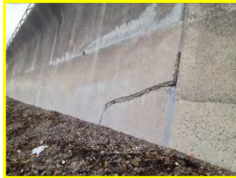
Incomplete or failed crack repairs on face of seawall (/1001c03).
