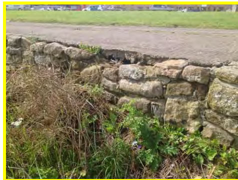
Some localised cracking and missing stones in masonry wall (/3001c09).
