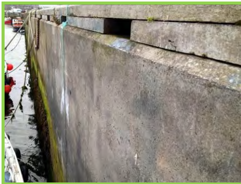
Slight bulge in quay wall adjacent to lifeboat station not observed (/3001c05).
