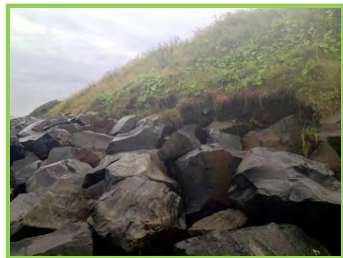
Minor erosion and cliffing of earth cliffs behind crest at north end (/3901c05).
