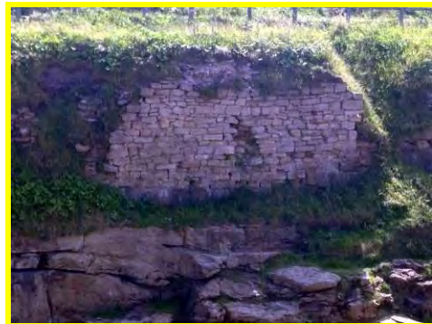
Gaps and missing blocks at the east end of the wall (/401c07).
