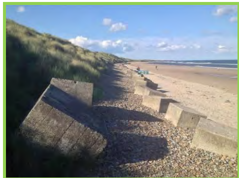
Dunes at north end of Druridge Bay protected by cobble berm and concrete blocks (/3201c15).
