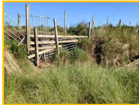
Breach in the embankment at south end of revetment (/1401c27).
