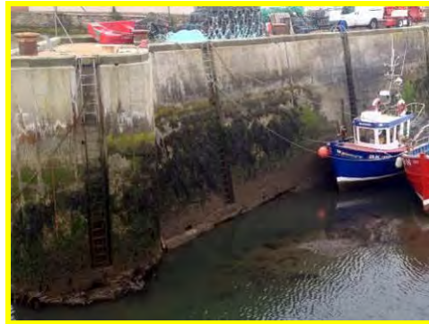
Some evidence of undermining seaward end of South Pier (/1701c14).
