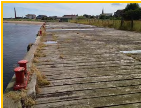
Low beach levels fronting Spittal Quay exposing masonry toe (/901C07).
