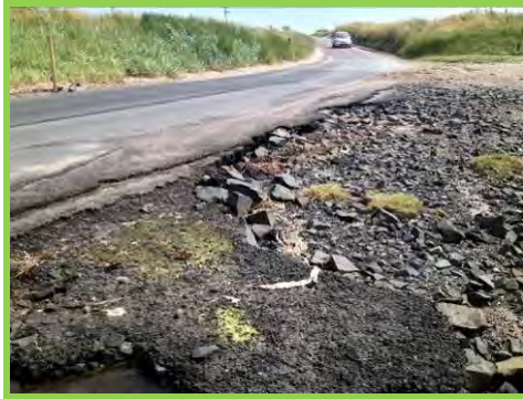
Localised erosion damage to road at Chare Ends (4901c01).
