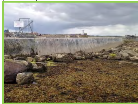
Repairs to crest of North Sunderland Harbour breakwater in good condition (/1701c21).
