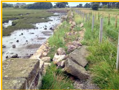
Collapse section of wall crest north of Peases Park and diversion of footpath (/2801c06).
