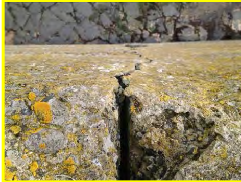
Full height crack on outside and inside face at seaward end of north pier (/2201c04).
