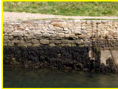
Settlement, abrasion and missing mortar in masonry quay wall (/4401c08).
