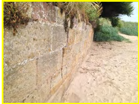
Vertical crack and some rotation in central section of wall (/2801c02).
