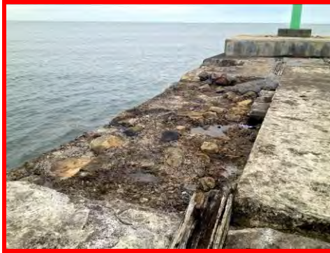
Loss of concrete deck slab at seaward end of North Pier.
