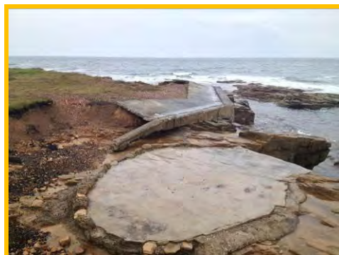
Undermining, outflanking and collapse of south end of low wall (3501c09).
