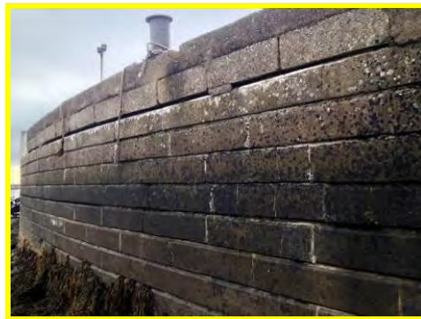
Missing mortar below coping (/4901c09).
