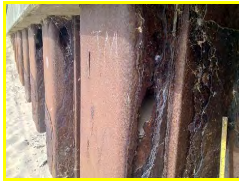
Corrosion of steel piles resulting in loss of section thickness and holes in the web (/4201c08).
