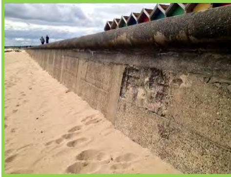
Areas of abrasion and exposed rebar on seawall adjacent to Links Road carpark (/4201c07).
