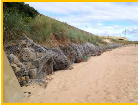
Deformed and burst gabions along the toe of the dunes at north end of South Beach (/4201c03).
