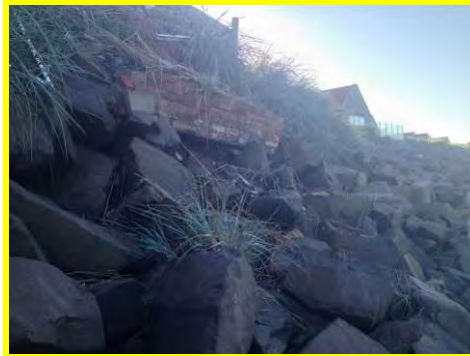
Erosion of earth slopes behind crest and tipping of building rubble (/3201c18).
