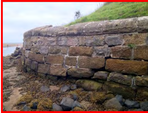
Cracks, loss of mortar and displaced blocks causing loss of material behind wall at Church Hill (/2801c13).
