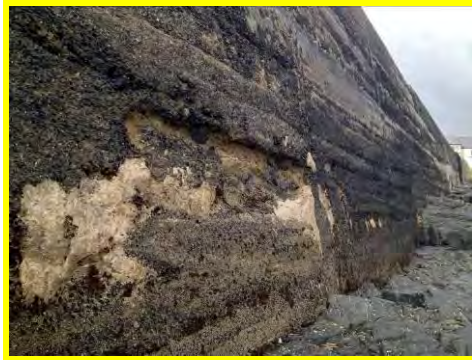
Abrasion to the seaward face of the north harbour arm at Craster (/2201c04).
