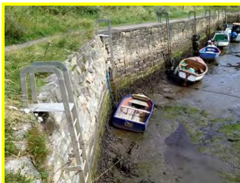
Some small gaps between blocks in wall along the inner north bank (/4401c05).
