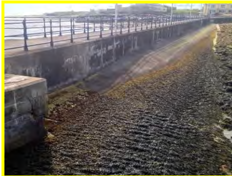
South Pier generally in fair condition with some abrasion and cracking evident (/3101c02).
