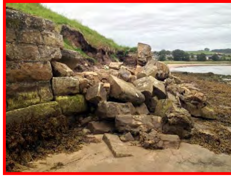
Collapse of section of wall due to loss of mortar, displaced blocks and loss of retained fill (/2801c13).
