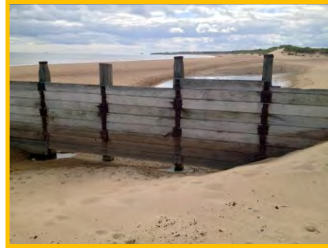
Scour beneath southern groyne due to re-alignment of Meggie's Burn (/4301c01).
