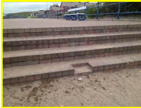
Missing blockwork surfacing on promenade steps (/1001c03).
