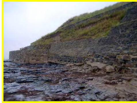
Cliff slumps at beach access ramp in 2012
