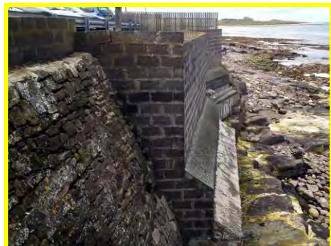
Missing mortar and gaps between upper masonry wall (/1701c03).
