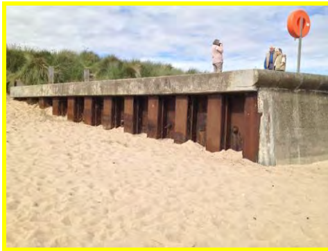
High beach levels in front of sheet pile return wall (/4201c08).
