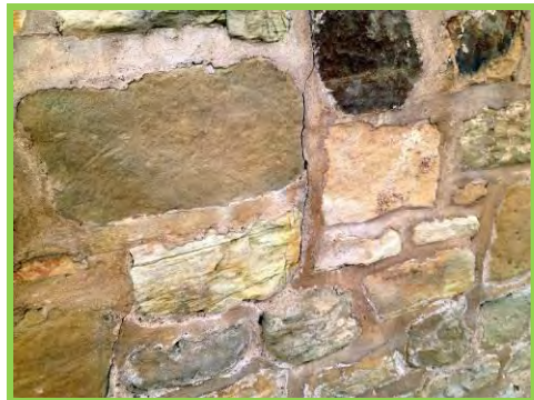
Minor cracks visible in masonry wall fronting the boat club (/2801c03).
