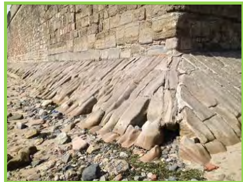
Historic abrasion to footing of seawall (/801c06).
