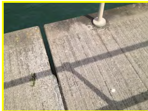
Minor movement in one deck section and loss of sealant (/3101c01).
