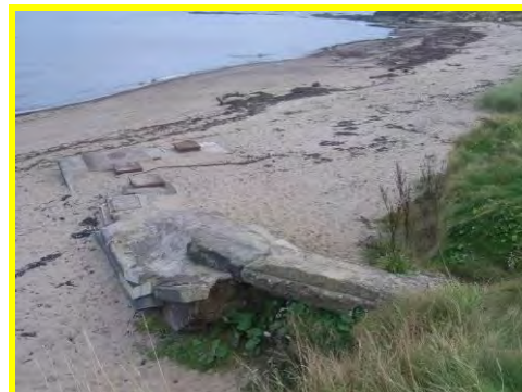
Dilapidated outfall requiring removal or repair (/3101c09).
