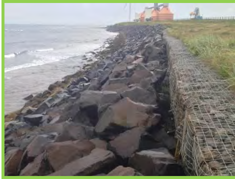
Some displacement of rocks at the toe of the revetment at North Blyth (/4001c01).
