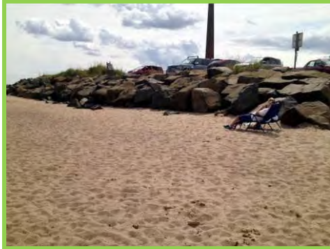
High beach levels at Sandstell Point burying the toe of the revetment (/901C10).
