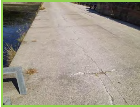
Minor cracking in old concrete deck slab (/701c14).
