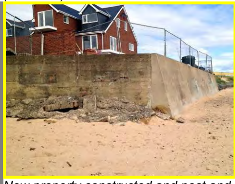
New property constructed and post and plank crest wall removed in 2014 (/4201c04).
