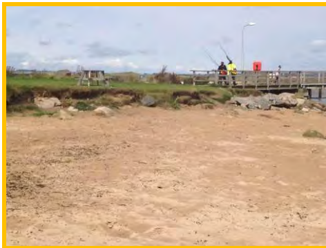
Continued erosion of low earth bank despite dumping of construction waste (/3001c07).
