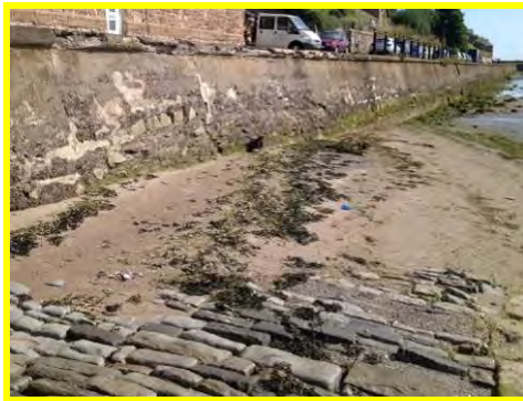
Damage to sections of coping along the Pier Road masonry seawall and displacement of cobble stones on the slipway (/801c07).
