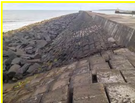
Rock armour on north side of pier in good condition, some gaps visible in blockwork (/3001c01).
