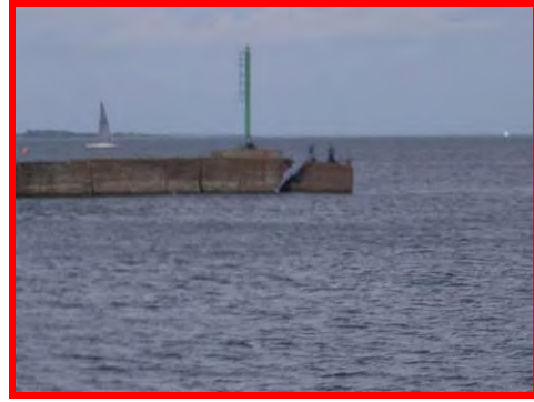
Large crack and rotation of tip of North Pier.
