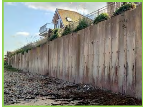
Minor signs of cracking and rust staining to concrete seawall (/1701c31).
