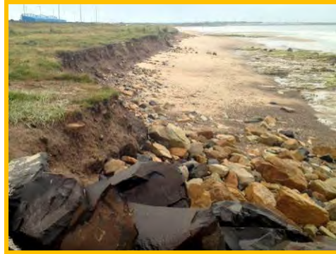
Erosion and outflanking at the north end and placement of smaller armour rocks (/4001c01).
