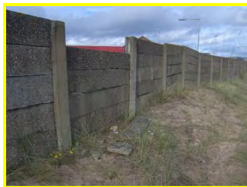
Some broken and missing planks along wall at back of dunes (/4201c11).
