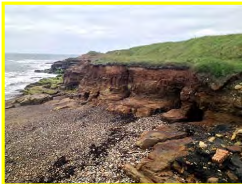
Ongoing erosion in thin layer of overlying soft material at Beacon Point (/3501C03).
