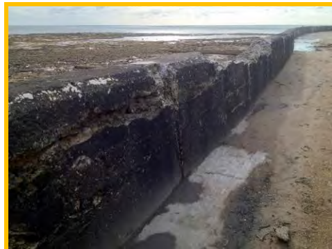
Significant horizontal cracking and spalling of crest wall (/4001c04).
