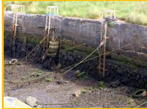
Coping at east end of wall cracked and highly abraded with large gaps and some missing blocks at the toe (/4401c06).
