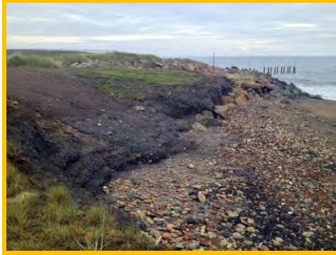
Erosion and onset of outflanking at south end of revetment (/3401c08).
