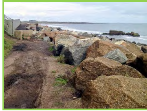
Minor erosion behind crest of revetment fronting power station (/3401c08).
