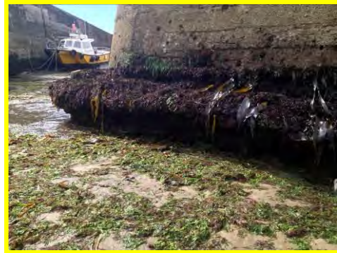
Initial undermining of toe apron at seaward end of north pier (/2201c04).
