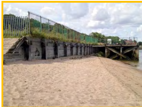
Displacement of stones and unravelling of masonry toe at Spittal Quay (/901C07).
