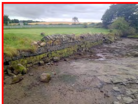
Significant collapse of central section of blockwork wall at Warren Mill (/1501c02).
