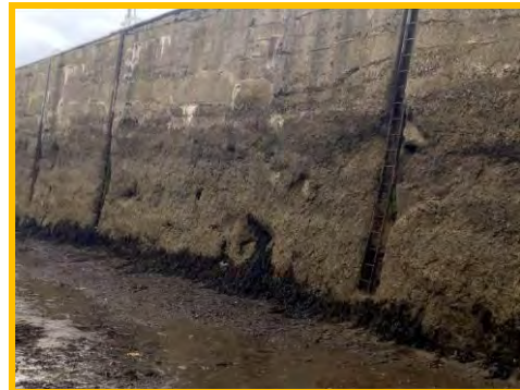
Significant abrasion, holes and small voids in inner face of Pier (/1701c09).
