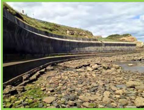
Slips in soft cliffs above seawall and material falling onto foreshore (/4401c14).
