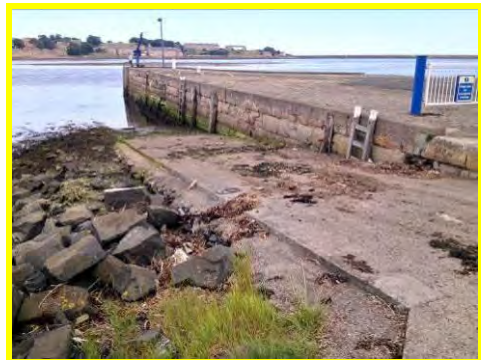
Abrasion and cracking of masonry blocks on west face of Spittal Pier (/901C06).
