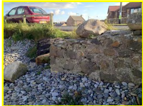
Loose coping stones at south end of seawall at Beadnell (/1701c37).
