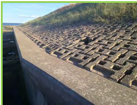
Missing block along concrete revetment at south end of Cresswell (/3201c19).
