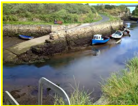
Some missing blocks and rotation of outer wall of slipway (/4401c05).
