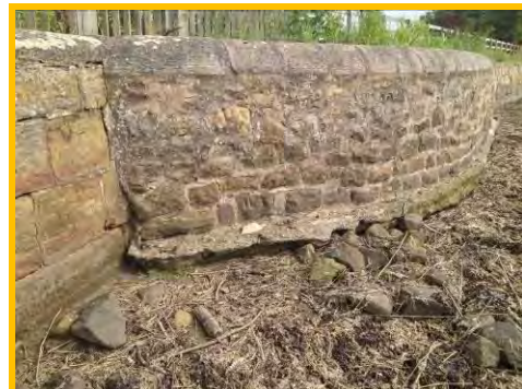
Initial undermining along one section of wall (/2801c10).
