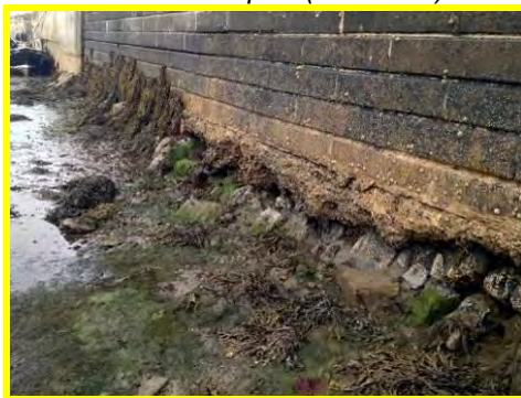
Undermining and voids at toe of northern face of pier (/4901c09).
