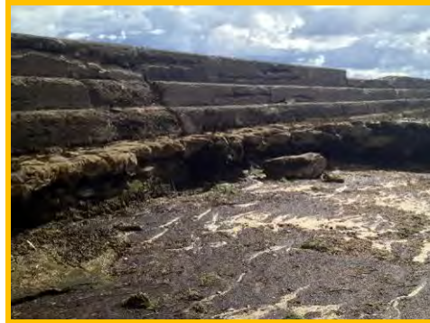
Cracking, spalling and undercutting of the rock foundation (/701c04).
