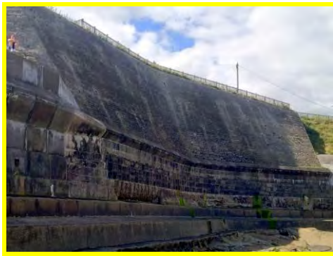
Loss of mortar on the recurve along most of the wall (/4401c15).
