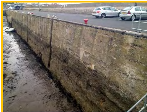
Significant abrasion, holes and small voids in inner face of Pier (/1701c09).
