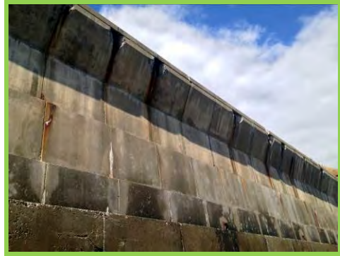
Spalling of concrete along upper section of seawall at north end of Collywell Bay (/4401c14).
