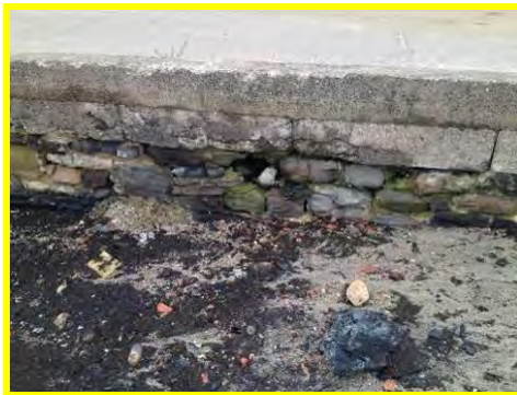
Missing mortar and voids in masonry section of harbour pier (/4901c09).
