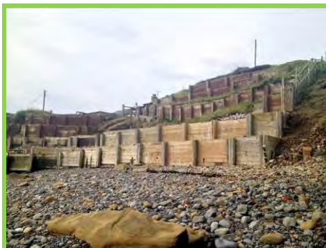
Erosion and slips at the northern edge of retaining wall could lead to outflanking (/3301c01).
