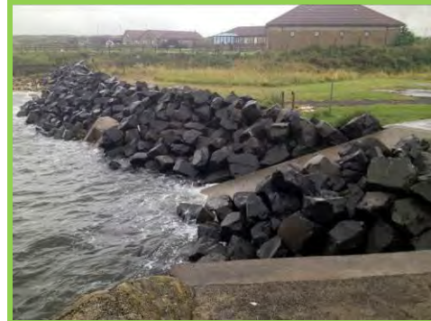
Slipway Slight undermining and outflanking of old concrete outfall at Spital Point (/3601c11).
