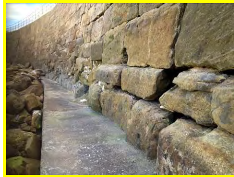
Gaps and some larger holes between blocks in masonry seawall (/4401c11).
