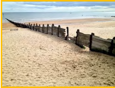
Gaps between groyne planks, arson damage and low beach levels (/4301c01).
