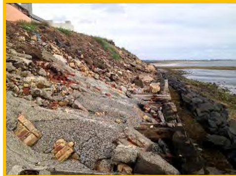
Erosion of slopes behind timber breastwork and dumped construction waste (/4001c03).
