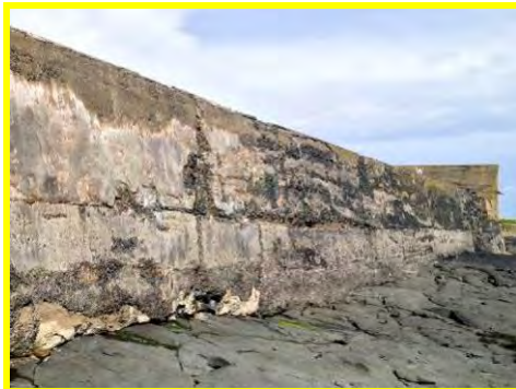
Abrasion and vertical cracks to outer face of south pier (/2201c11).
