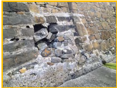
Missing blocks resulting in a deep hole and void behind (/1701c36).
