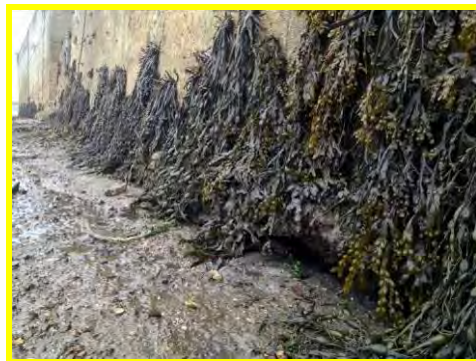
Undermining and voids at toe of northern face of pier (/4901c09).
