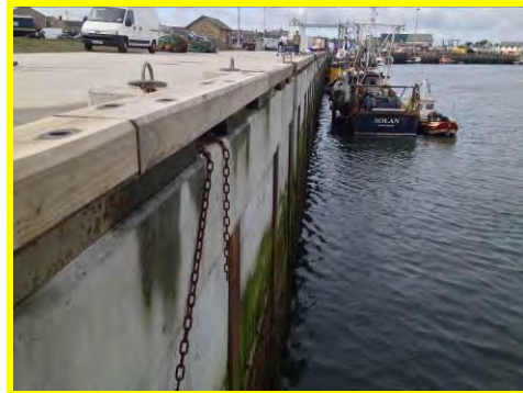
Repairs to failed section of Broom Hill quay completed in April 2013 (/3001c05).
