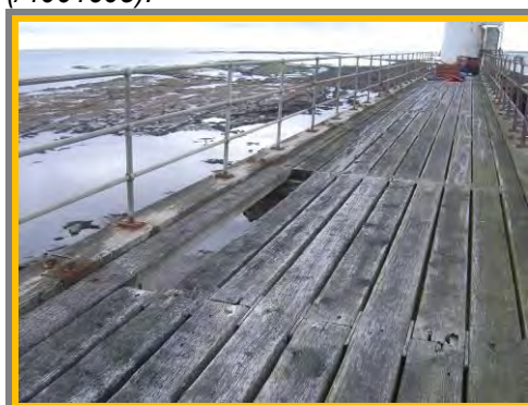
Missing sections of timber decking and rot at some fixings in 2012.
