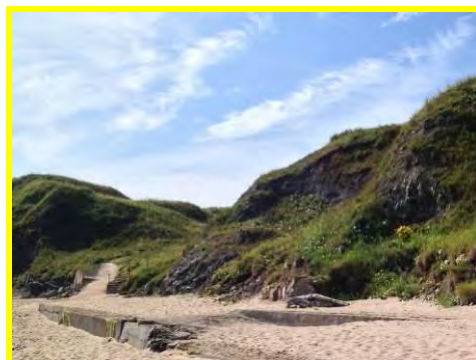
Concrete apron in poor condition, slumps in upper soft cliffs cutting back to footpath above (/701c07).
