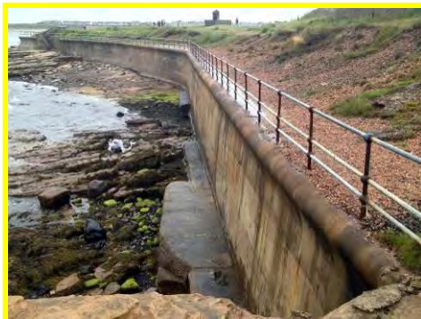
Erosion of the vegetated slope behind the crest of the seawall at Church Point (/3601c12).
