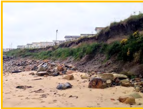
Active erosion in cliffs fronting north end of Newbiggin Caravan Park (/3501C05).
