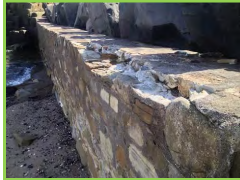
Damage to masonry along crest of low masonry wall at Wellhaugh Point (/3101c10).
