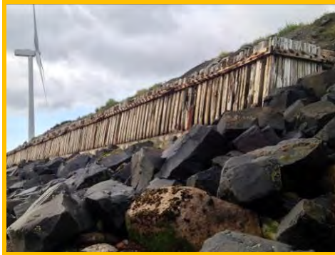
Broken and missing timber boards and rotten wailing beam to breastwork (/4001c03)
