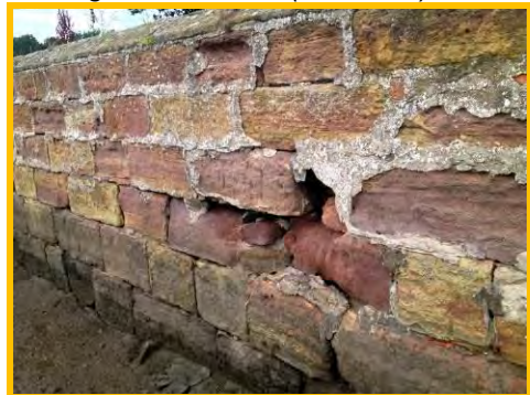
General abrasion, missing mortar and gaps along much of wall at Peases Pk (/2801c06).
