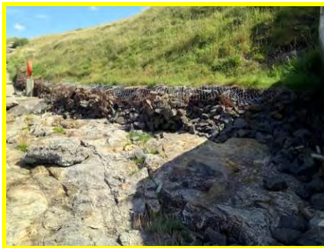
Gabion baskets at the bottom of the access ramp continue to degrade (/4401c19).
