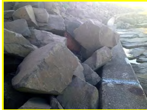
Erosion of earth slopes behind crest and tipping of building rubble (/3201c18).
