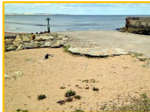
Undermining of concrete deck adjacent to groyne (/4402c02).
