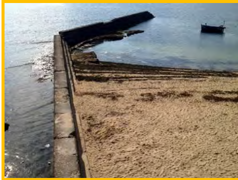
Damage to crest and head of Green's Haven Breakwater (/701c04).
