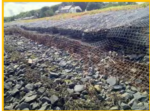
Loss of stone from the lower gabion baskets (/901c04).
