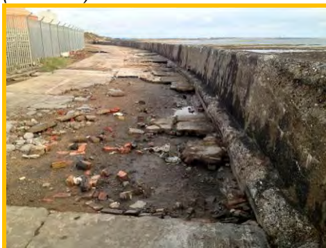
Breakup of concrete deck behind crest wall (/4001c04).
