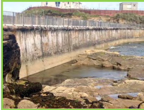
Localised cracks, rust staining and spalling along the wave wall (/3101c05).
