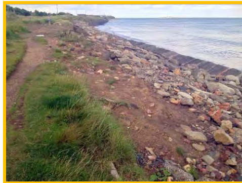
Erosion of low earth bank and dumped construction waste at Hauxley Nature Reserve (/3201c04).
