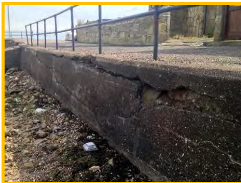
Horizontal cracks along the cope of the seawall at Bay View Road (/300c10).
