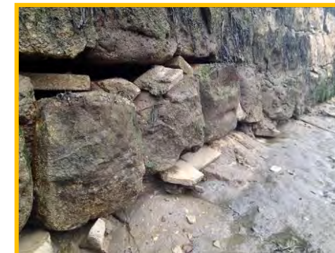
Localised undermining at the north quay resulting in movement of some blocks (/1701c52).
