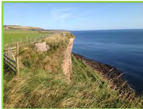
Sections of abandoned masonry wall and new fencing at north end of Marshall Meadows Bay (/601c01).
