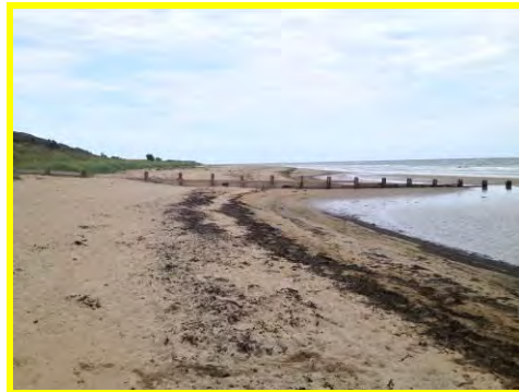
Groynes in poor condition and high beach levels south of Marsden Rocks (/2701c05).
