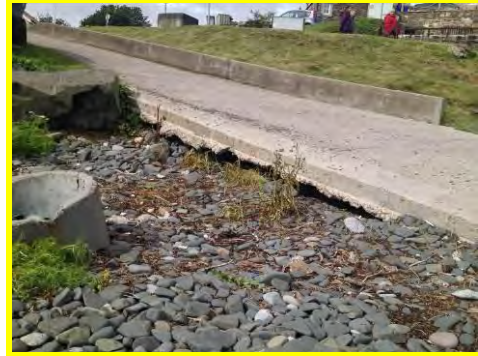
Undermining and a deep void beneath the boat ramp at back of harbour (/2201c06).
