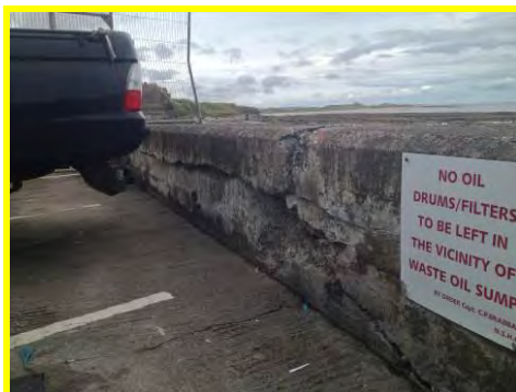
Significant horizontal crack in crest of seawall opposite RNLI building (/1701c06).
