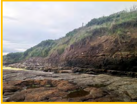
Erosion of toe of soft cliffs at Snab Point (/3301c01).
