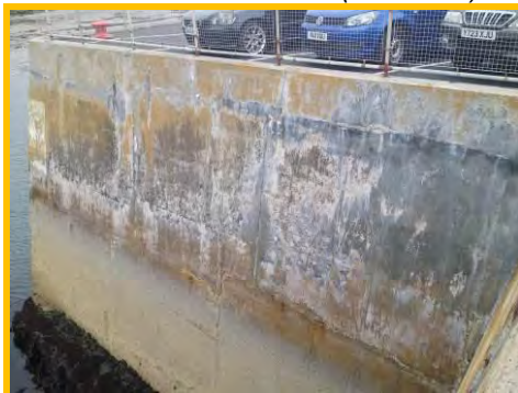
Large scour hole reported beneath Main Pier stub (/1701c08).
