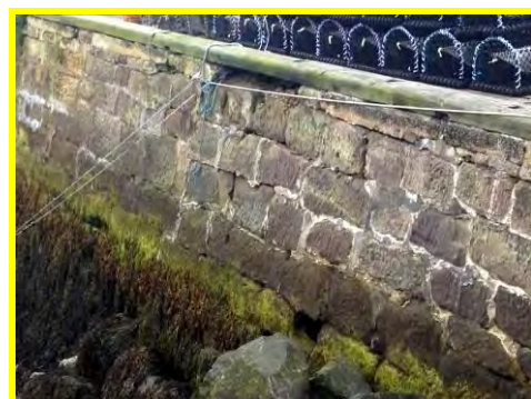
Some gaps beneath crest of Central Pier (/1701c10).
