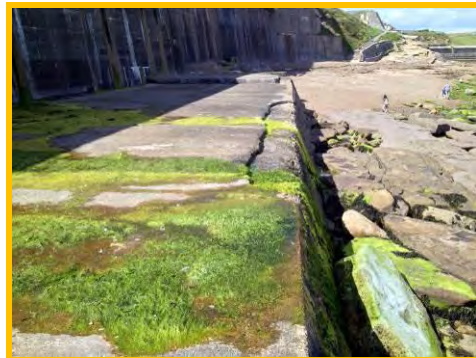
Significant abrasion at the toe and horizontal cracks (/4401c17).
