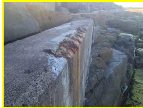
Incomplete crack repair resulting in corrosion and rust staining (/3201c18).
