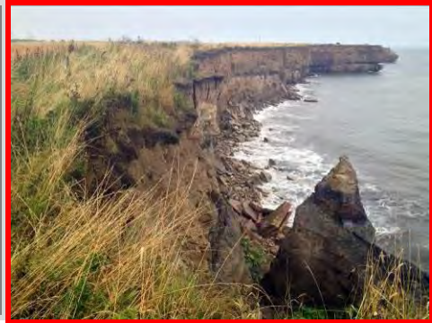
Partially collapsed cliff and closed footpath at Hawk Cliffs in 2014 (/3701c02).
