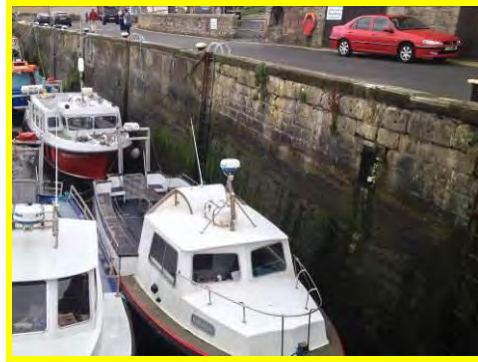
Some weathering of masonry blocks and loss of mortar (/1701c13).
