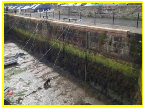
Some gaps between masonry blocks, timber edging protecting the cope (/3001c06).
