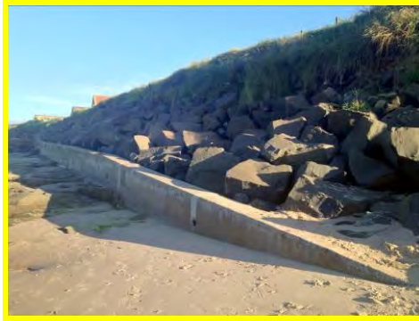
Lower beach levels fronting low concrete wall at Cresswell (/3201c18).
