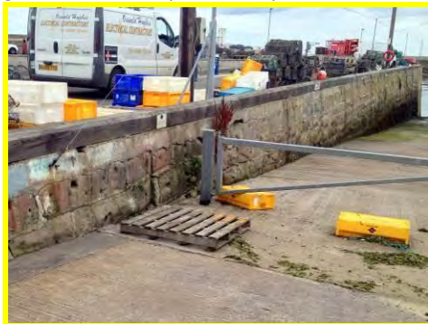
General weathering and missing mortar of blocks along outer face of South Pier (/1701c14).
