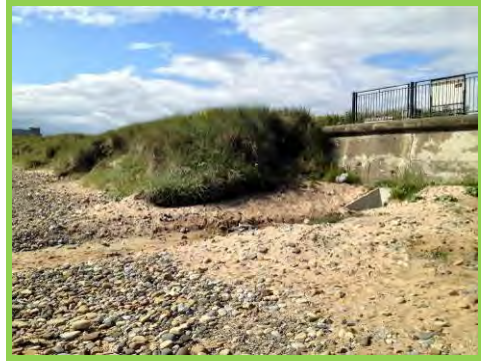
Localised erosion to the dune edge from the outfall constructed in 2009/10 (/4201c05).
