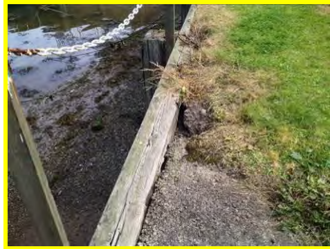
Displacement of stones and unravelling of masonry toe at Spittal Quay (/901C07).
