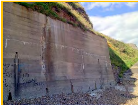
Notable vertical crack in high seawall at centre of the bay (/4401c17).
