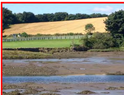
Significant collapse of central section of blockwork wall at Warren Mill (/1501c02).
