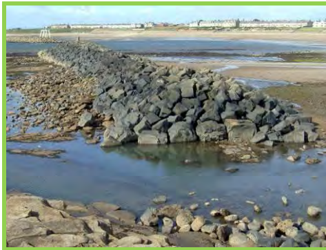
Displaced rocks along seaward side of north breakwater in Newbiggin Bay (/3601c14).
