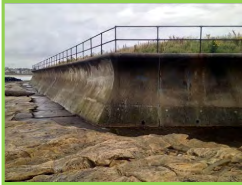
Some minor undermining of the toe apron of the recurved seawall (/3601c13).
