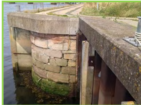
Loss of mortar between blocks in short section of masonry wall (/801c03).
