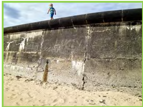
Cracks and staining in the seawall adjacent to the Dave Stephens Centre (/4201c06).
