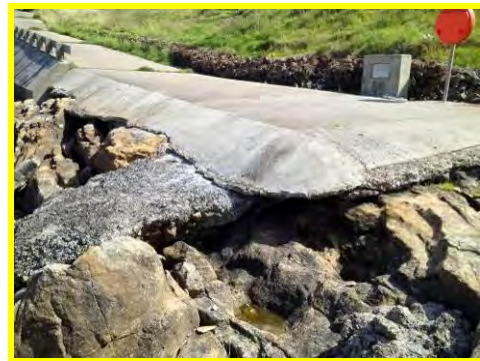
Undermining of concrete access ramp (/4401c19).
