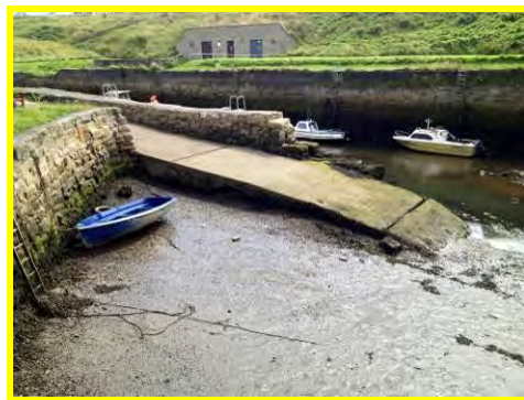
Full width cracks at top and bottom of slipway ramp (/4401c05).
