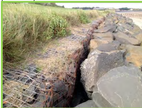
Localised erosion of embankment behind revetment crest (/1001c01).
