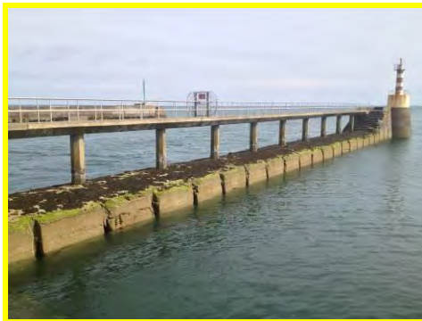
Significant abrasion to the base of the South Pier Head (/3101c01).
