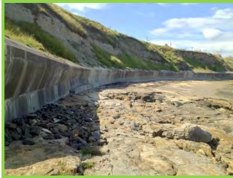
Slips in upper earth slopes and material on the foreshore at the south end of the bay (/4401c18).
