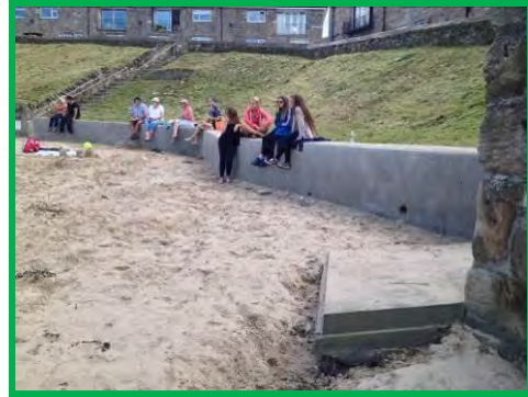
Onset of undermining of bottom landing of steps at low concrete seawall (/1701c16).
