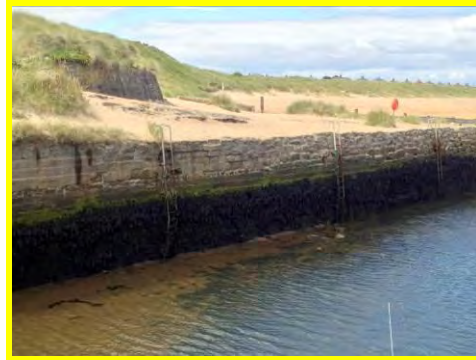
Accumulation of sand along crest of masonry wall on west side of entrance (/4401c04).
