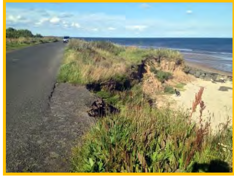
Cut back of the low earth cliffs close to the road at Hadston Scaurs slipway (/3201c14).
