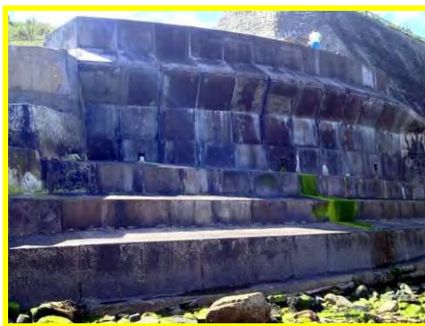
Missing flap valves and calcium deposits blocking southerly weep hole (/4401c16).
