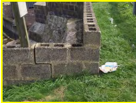
Settlement of fill and rotation of crest wall (/1701c03).
