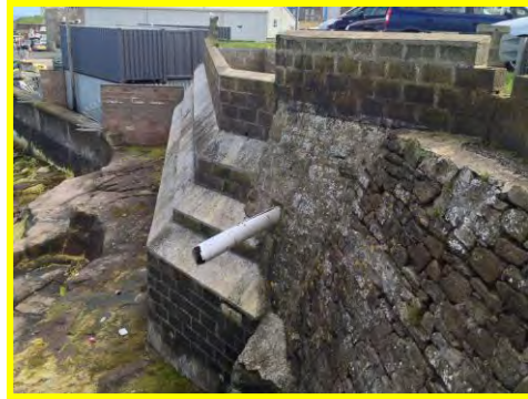
Missing concrete coping blocks along part of toe (/1701c02).
