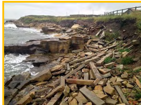
Erosion of soft cliffs continues despite tipping of building/quarry waste (/3701c01).
