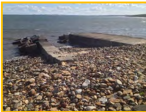
Abrasion of blocks, broken concrete and missing flap valve cover to outfall (/3201c09).
