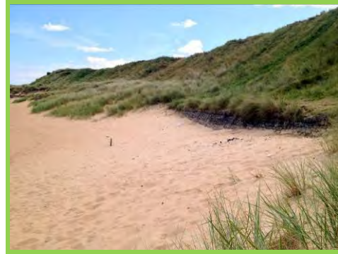
High beach levels and vegetation burying masonry wall north of harbour (/4401c01).
