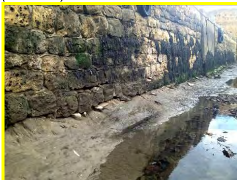
Localised undermining at the north quay resulting in movement of some blocks (/1701c52).
