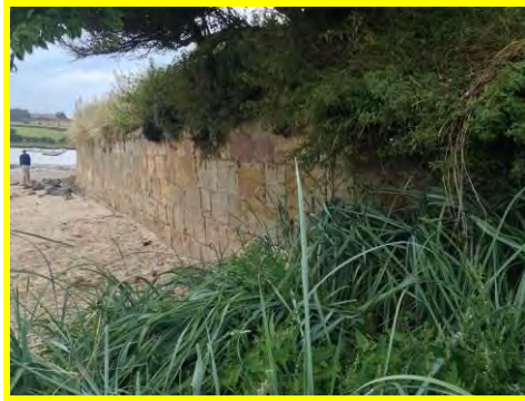
Stable beach levels and vegetation growth fronting the wall at Riverside Road (/2801c02).
