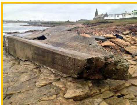
Damage to crest slab and undermining of the low wall at Newbiggin Point (3501c09).
