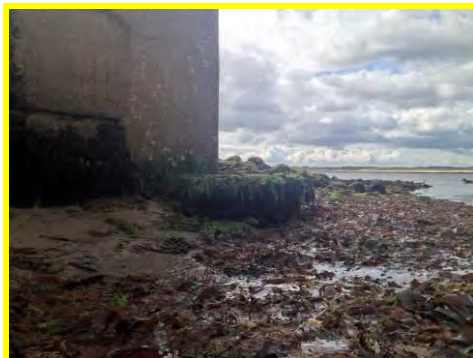
Undercutting of the toe apron at the head of Beadnell Harbour breakwater (/1701c50).
