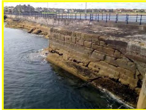
Abrasion and cracking of the South Pier at the junction with Bay View Road (/3101c02).
