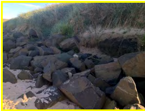
Loosely placed rock and localised crest erosion south of Cresswell access steps (/3201c17).
